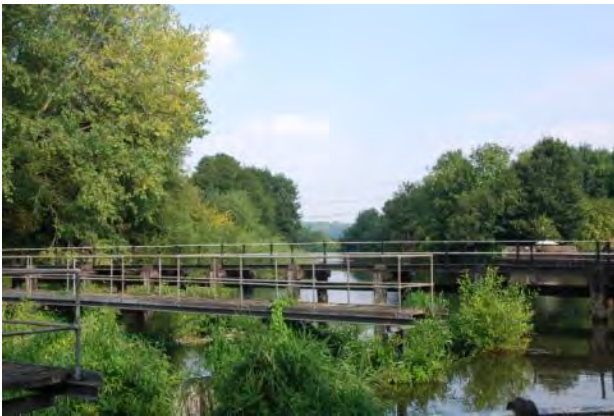
Local industrial heritage foci are provided by sites such as Dobb's Weir
