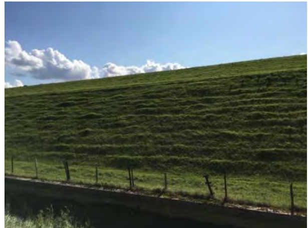
Sheep trails on steep reservoir embankment.
